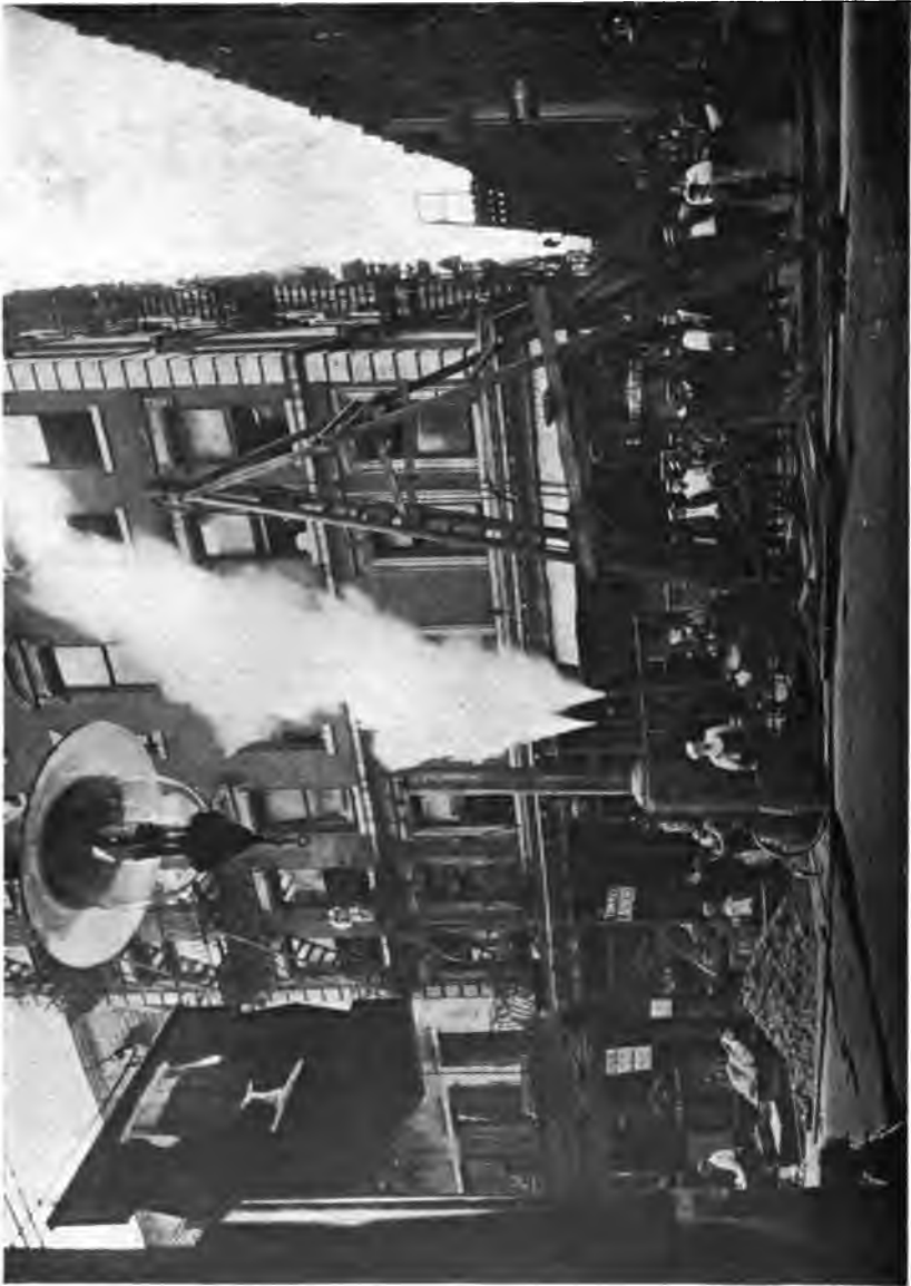
PLATE 21.—Minnesota Diamond Drilling Rig in New York City. Drilling in rock for core.
